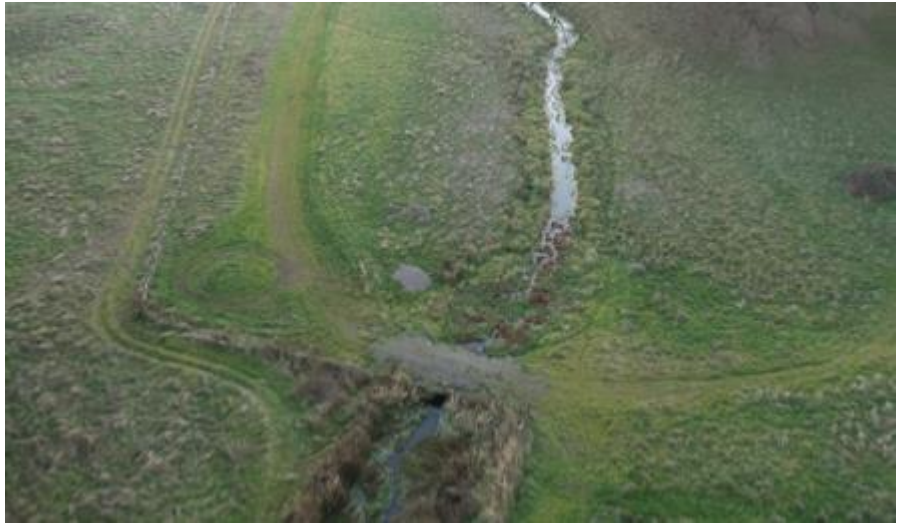
A south facing aerial view of the upstream culvert on Marion Creek. The culvert provides legal access from the property gate on Marion Road to the habitats found west of Marion Creek.
